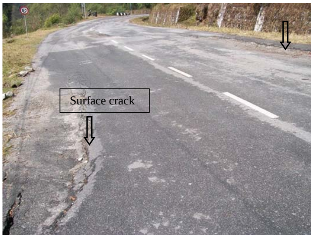
Fig. 3 Road damage due to landslide at Bulbulay road, Gangtok
