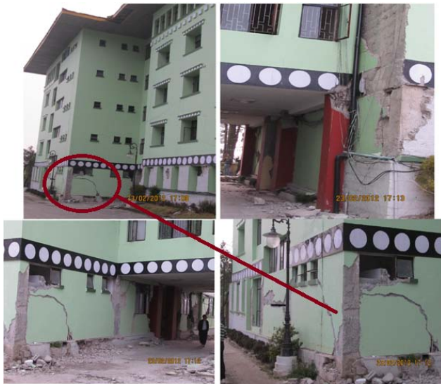
Fig. 8 Photos of damaged secretariat building
