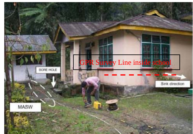
Fig. 6 Distressed School Building at Upper Dzongu
